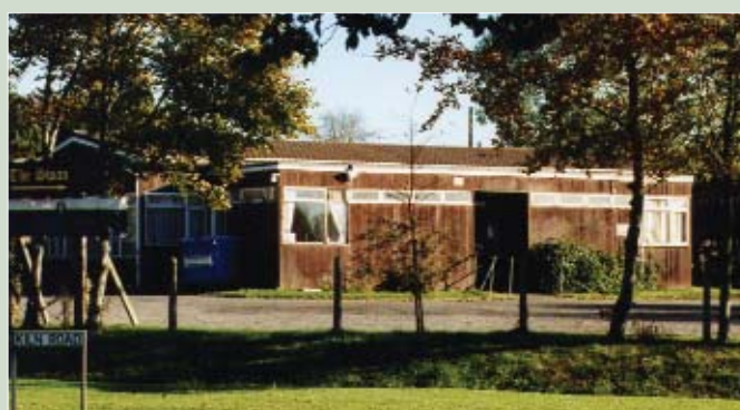
The delapidated Village Hall
